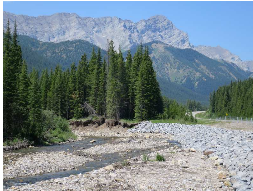
Repair of the Highwood River (1870m) after the 2013 flood below the Elk Range (2750m)
